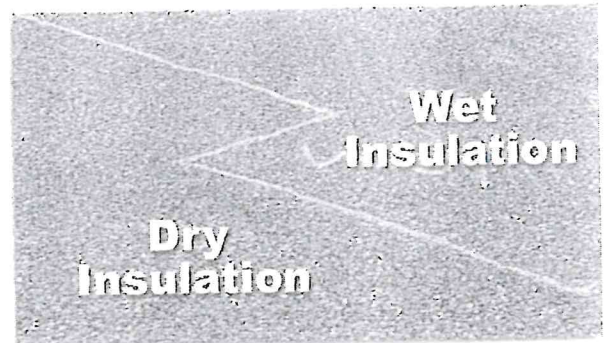
Control image, wet sections marked for removal
